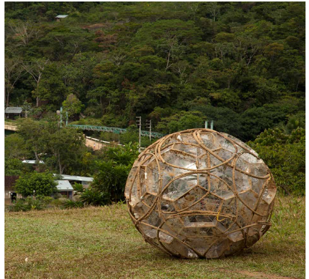
Fig. 1. Spherical structure completed (including internal mechanism), ready to be plastered with quincha paste. San Roque de Cumbaza, Peru. Summer 2013. Photo: Alejandro Borsani.
