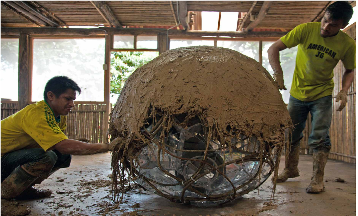
Fig. 2. Local builders Adriel Vasquez Saavedra and Regner Cachique Sangama plastering the external quincha skin. San Roque de Cumbaza, Peru. Summer 2013. Photo: Alejandro Borsani.
